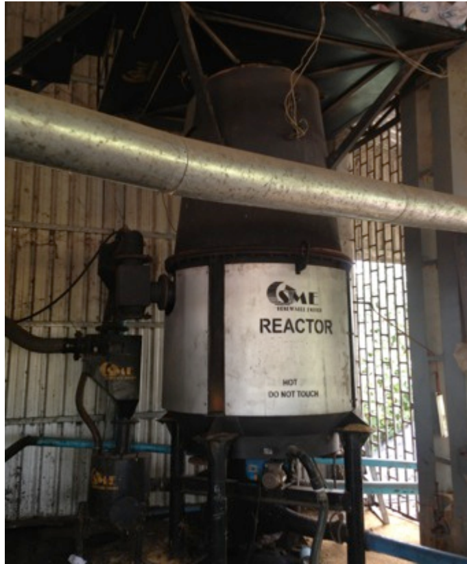
Figure 1. Ankur gasifier Ms. Savoeun's rice mill, Deum Pou village, Phnom Penh, Cambodia, 2014 - 12 - 19
