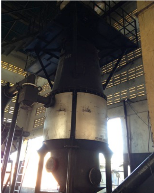
Figure 8: 150kW Ankur downdraft gasifier at UNIDO Project, Siem Siep Province, Cambodia, 2014-12-20
