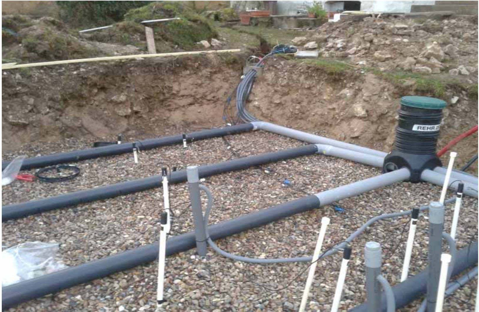
Pre-treated wastewater drains and the probes
